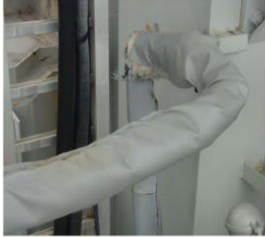
OLD MI cable insulation
