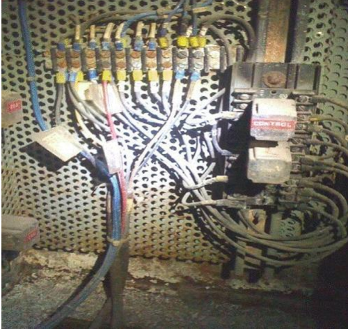
Corroded Freeze Protection Panel
