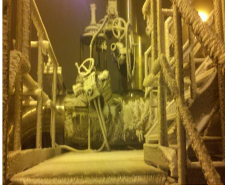
Access to equipment after the fact can be very difficult.
